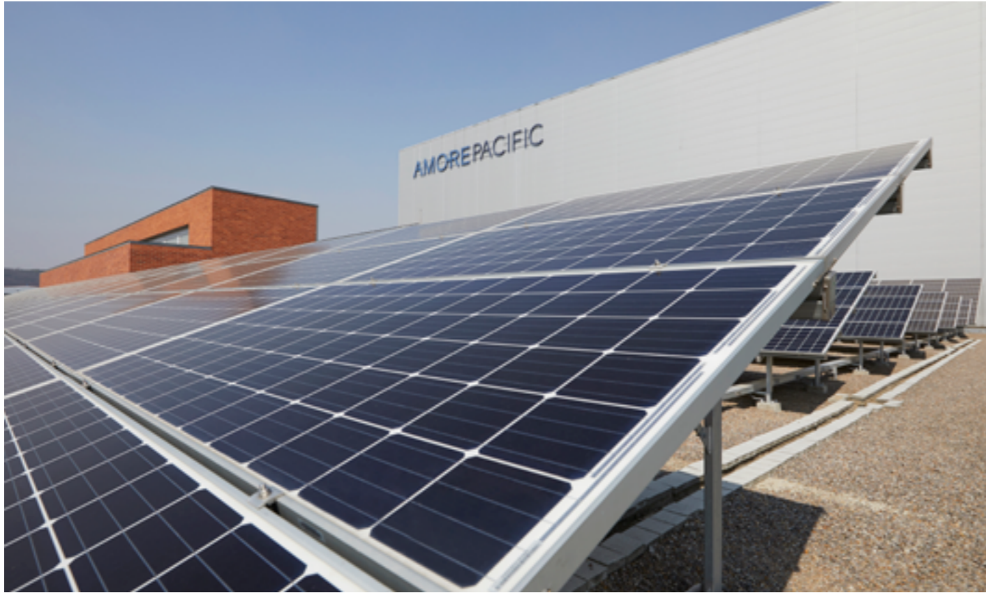
Photovoltaic panels at Osan Amore Beauty Park
